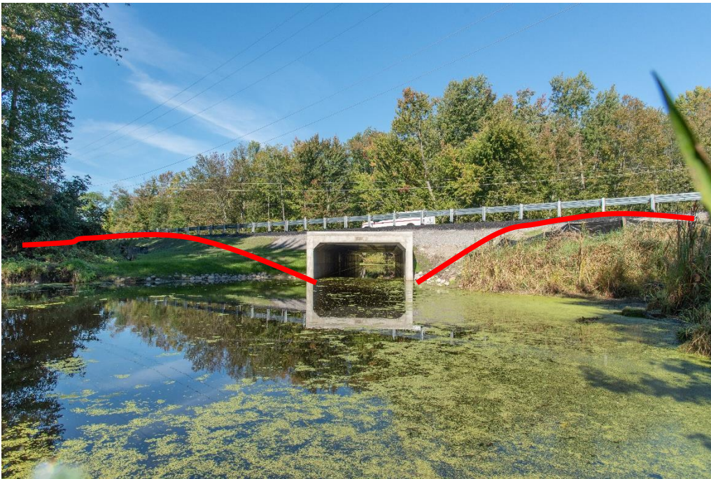
Image 6: New box culvert installed on Monck road at Sucker creek with red lines depicting placement of permanent exclusion fence. Note the culvert is large providing maximum visibility and openness through the length of the structure. Photo Credit: Toby Rowland.
