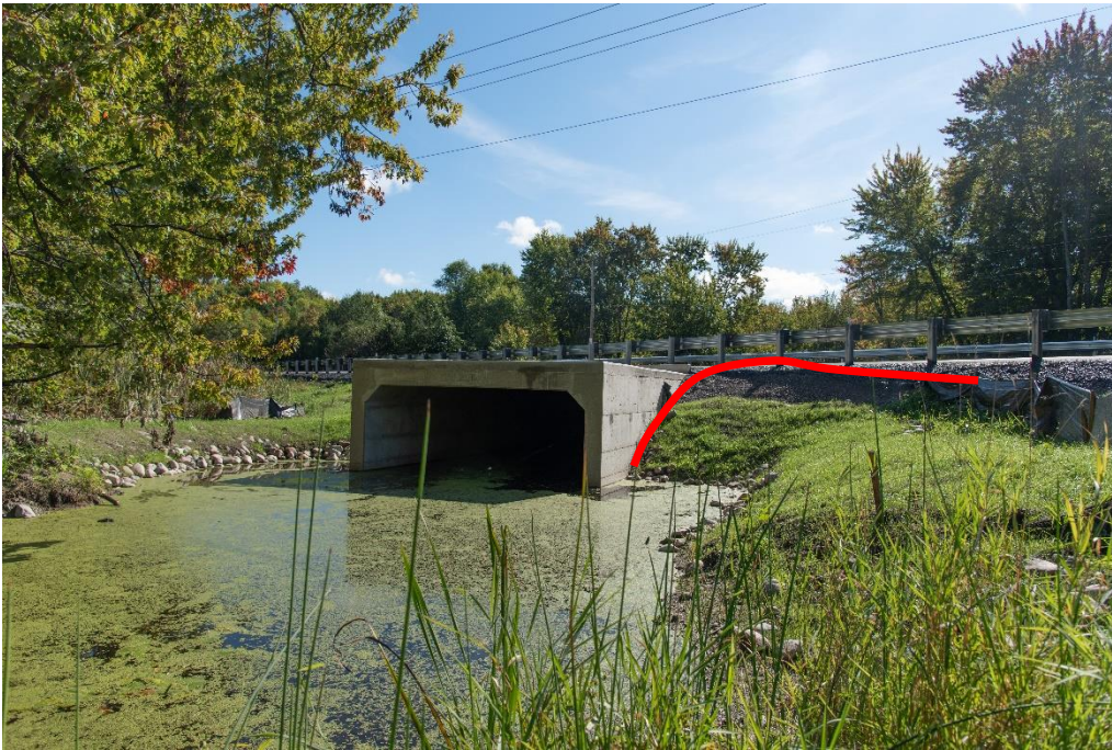
Image 7: New box culvert installed on Monck road at Sucker creek with red lines depicting placement of permanent exclusion fence that will abut the drainage culvert to funnel animals to the entrance. Photo Credit: Toby Rowland.
