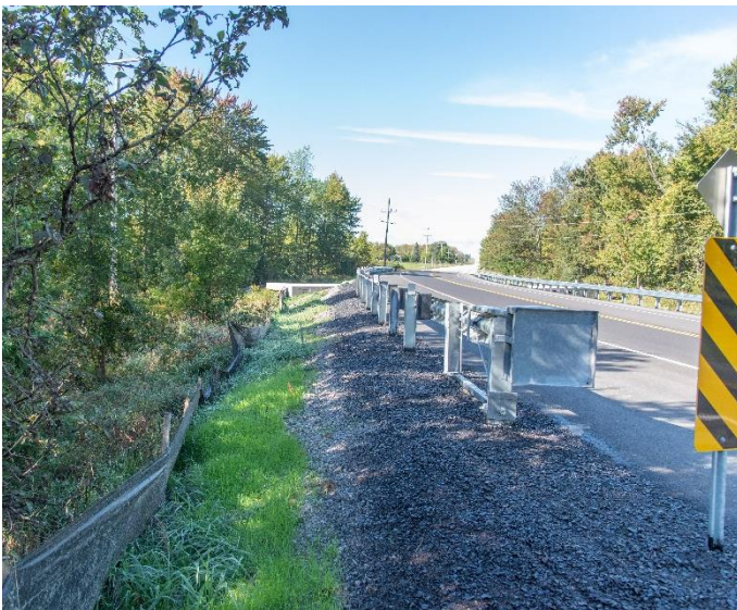
Image 8: Silt fence along the road corridor that needs to be replaced with more permanent exclusion fence. Note existing guard-rail that is ideal to protect exclusion fence from snow, and or could be used to attach exclusion fence onto the structure. Photo Credit: Toby Rowland.
