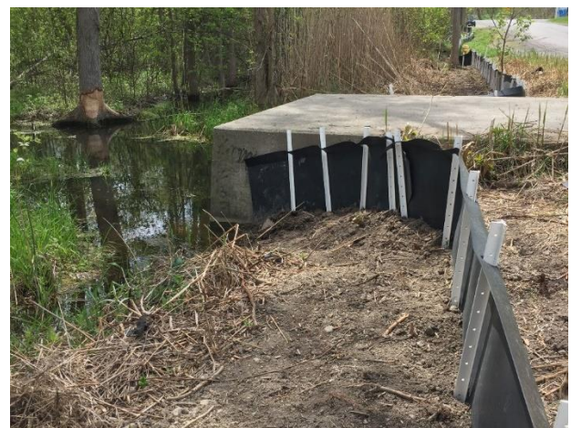
Image 9: Example of exclusion fence abutting a large drainage culvert on the Scarborough-Pickering Townline road in Rouge Urban National Park. Photo Credit: Paul Yanuzzi.
