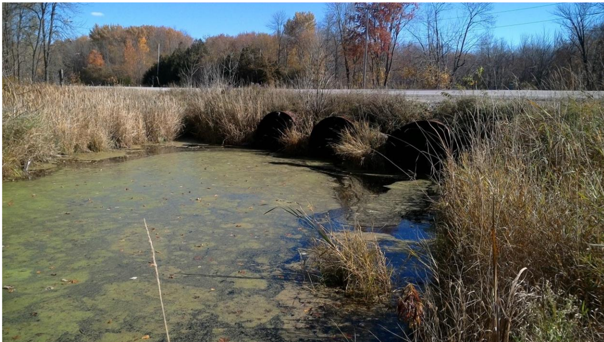
Image 4: The three 1800 mm steel culverts that were replaced at Sucker Creek along Monck Road (Riverstone Environmental Solutions 2021).
